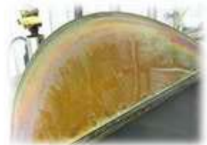
CIP Tank Lid Staining
